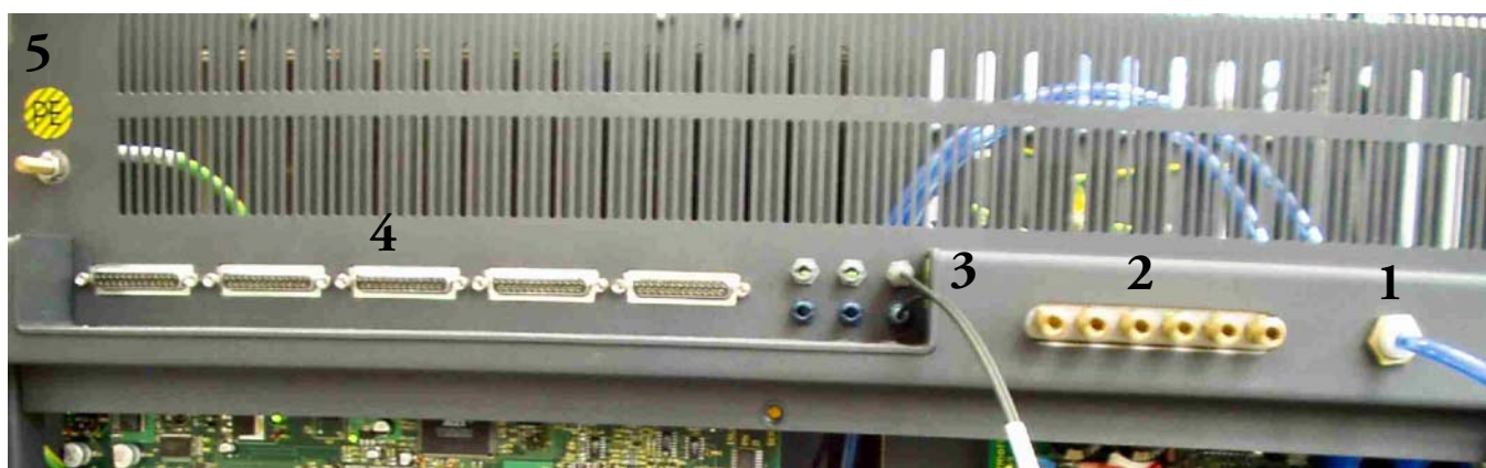
Figure 2-47. Electronics Cabinet - Upper Faceplate
