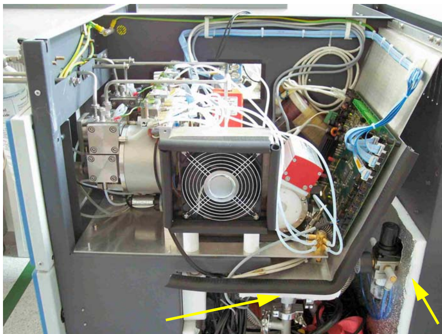
Figure 7-13. Thermal Insulation Mats and Chimney
