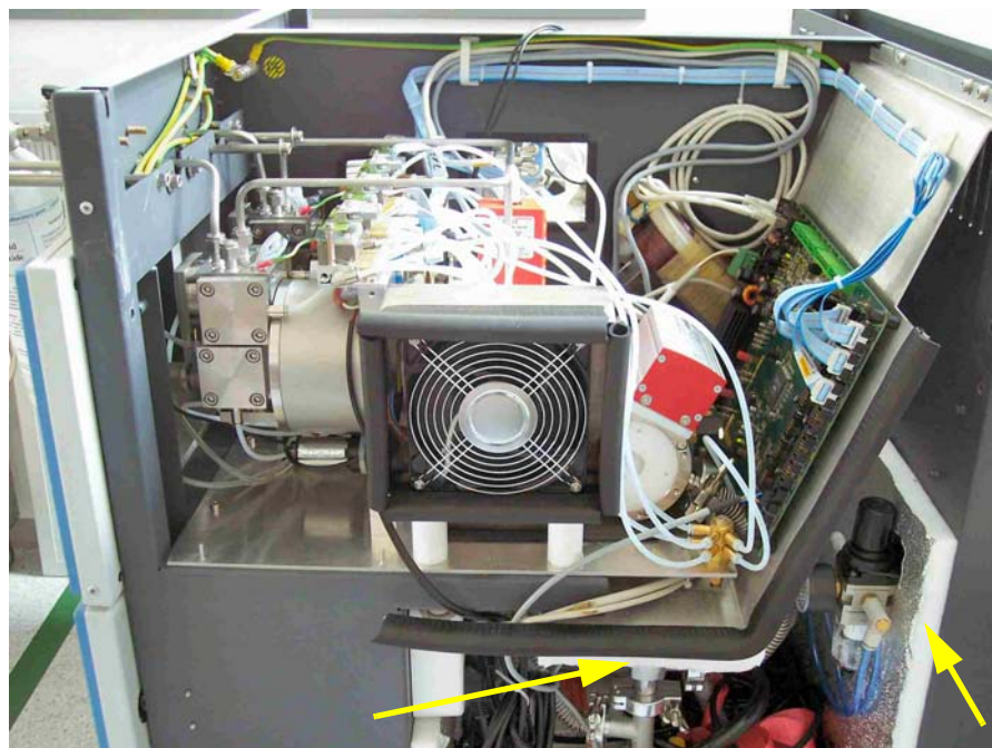
Figure 7-13. Thermal Insulation Mats and Chimney
