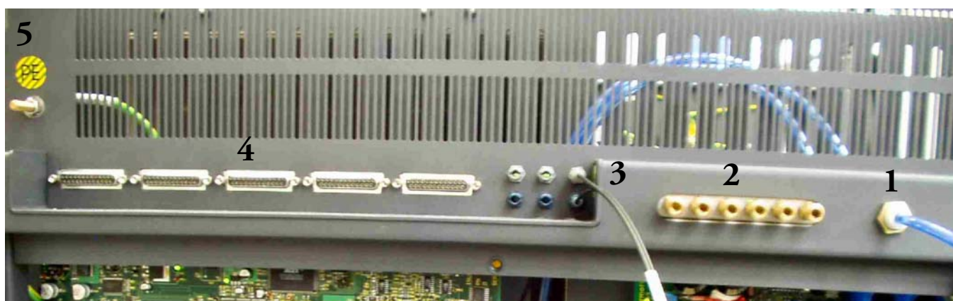
Figure 2-47. Electronics Cabinet - Upper Faceplate
