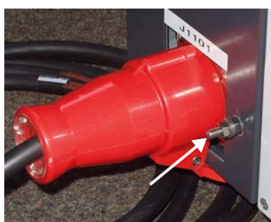
Figure 4-3. Grounding bolt right to main switch
