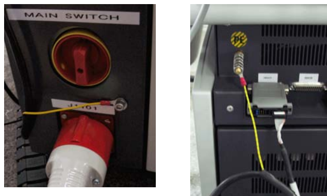
Figure 7-9. Grounding cable at MAT 253 (left) and DELTA series (right)
